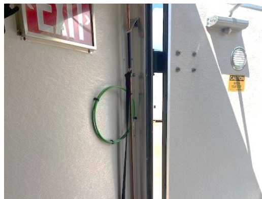
Ground Rod (Located left of Rear Entry/Exit Door)
